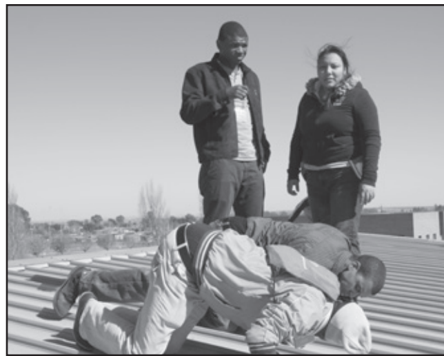
Tanya and Peter take measurements and locate the installation area for the solar panels on the IT building of Wilberforce Community College.
